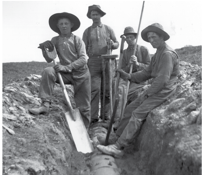
These tilters on the Sweet Farm near Franklin dug trenches that slanted downward and away from the field. In the trenches they laid cylindrical, clay drainage tiles. Rainwater drained through the soil, into the tiles, and was carried away from the field. Tilters usually used a grid system to organize the drainage across a field. Courtesy Illinois State Museum, photographer Leroy Sweet.
