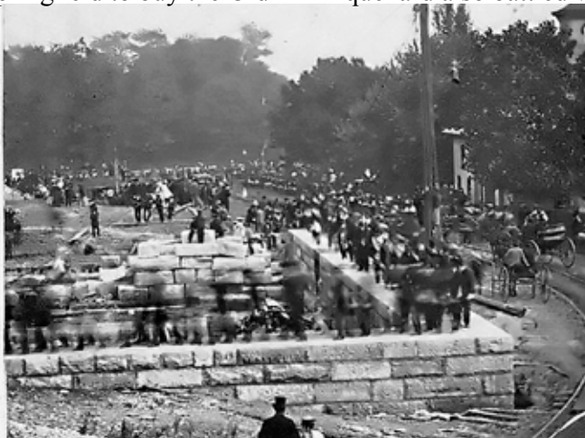
This April 14, 1871 photo shows the foundation of the Statehouse under construction. Photo courtesy of ilstatehouse.com
